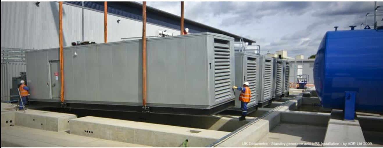
UK Datacentre - Standby generator and UPS Installation - by ADE Ltd 2009.
