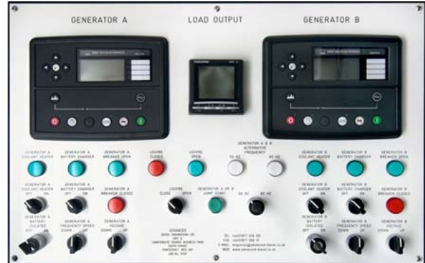
The Encore Duo main panel includes dual DS7510 control units.
