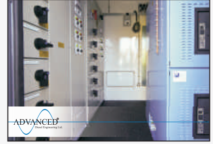
Switched distribution & interlocked change over
